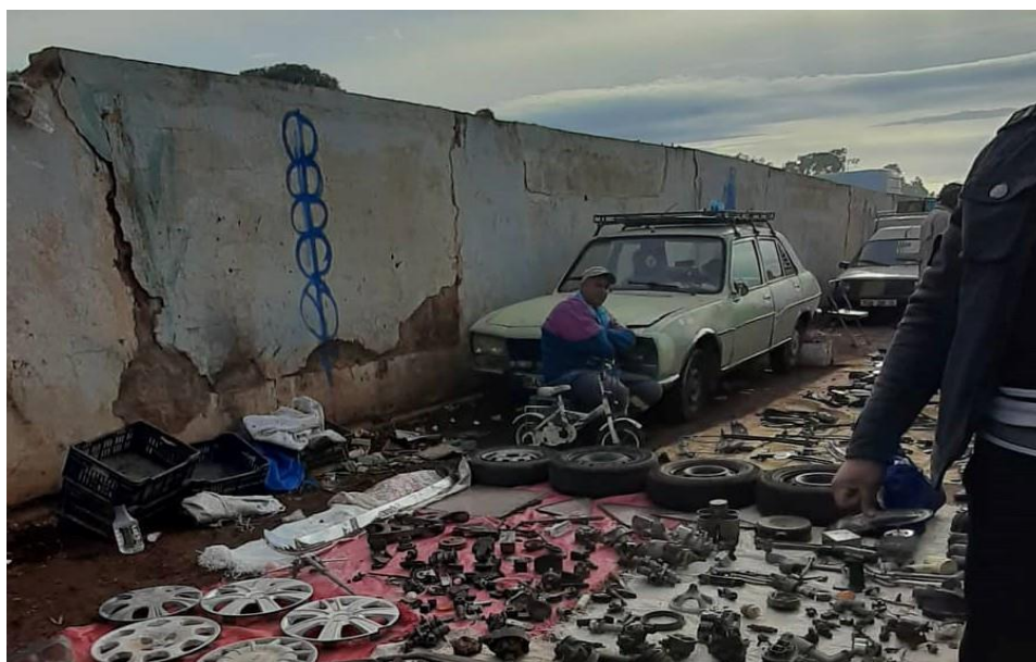
Photo 1-2: Fissuration du mur
